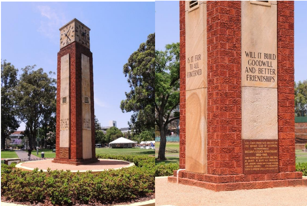
Figure 28: Detail of the Rotary clock tower showing the textured brick construction with inscribed sandstone panels. (Photos: C Betteridge, 2014)
