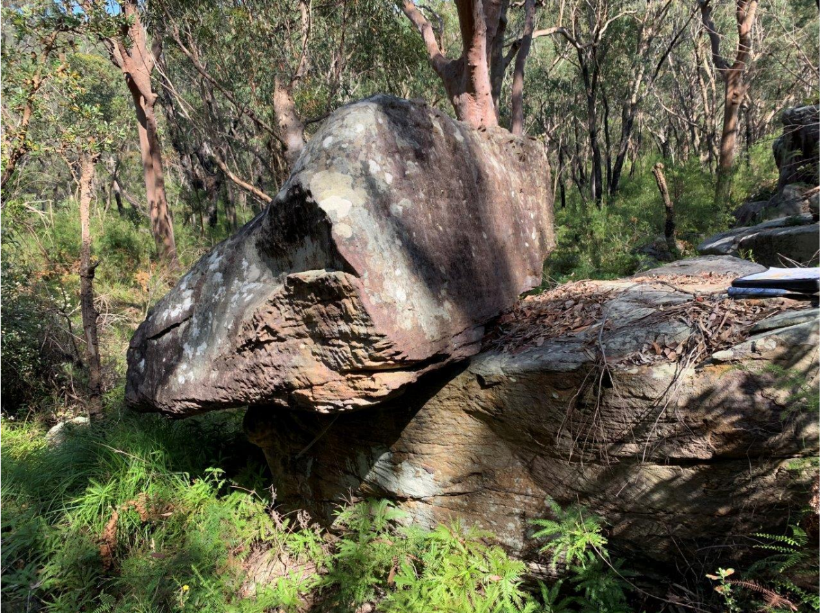
Photograph 9: View looking west of previous large failure
