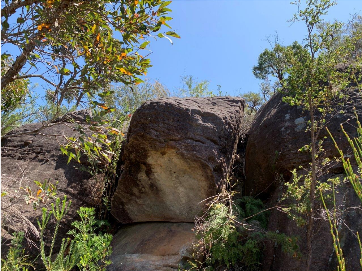
Photograph 5: View looking west, large loose block (~1m x 1.5m) at crest, potential slide failure
