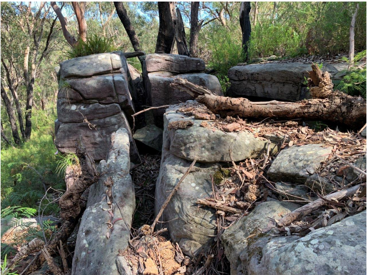
Photograph 12: View of large void approximately 0.35m wide and 1.3m deep, vegetation debris blocking truth depth
