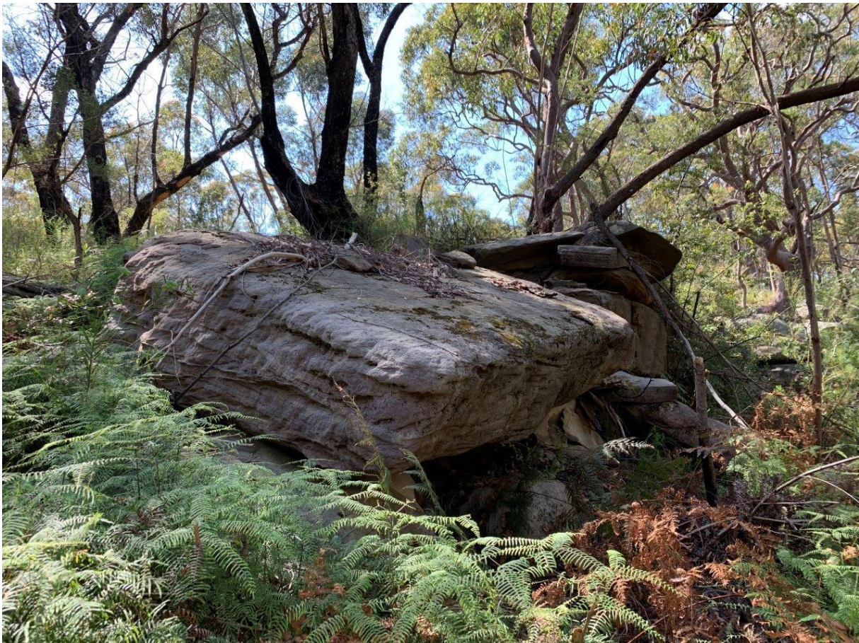
Photograph 20: View looking south-east, previous failure of large sandstone bed up to 1.5m thick
