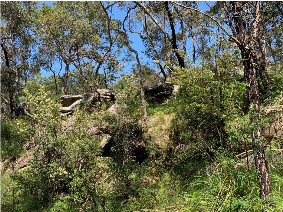
Photograph 4: View looking south towards slope crest, overhangs and loose blocks observed
