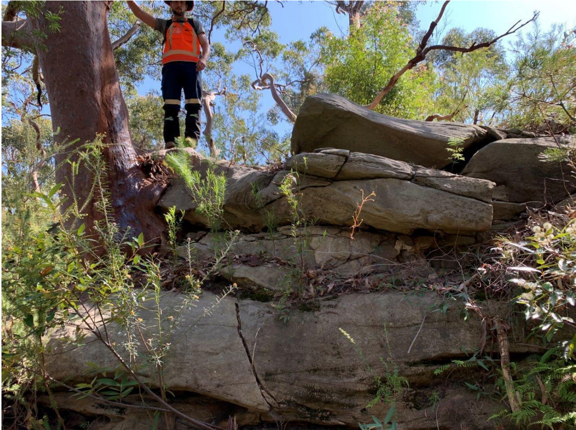
Photograph 17: View looking east, cracking observed within sandstone precipice, potential root jacking from mature tree
