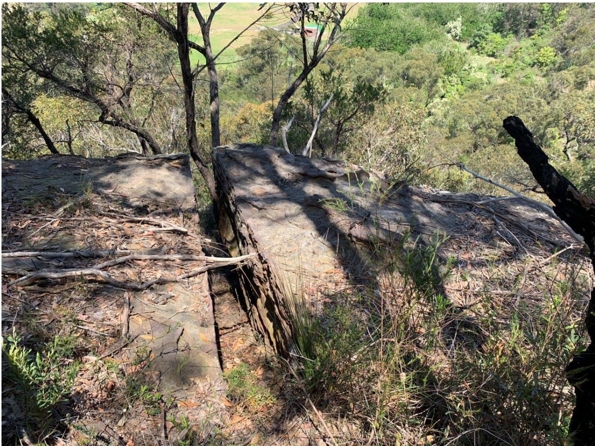
Photograph 6: View looking south at crest, open void ~0.3m with large overhanging blocks at crest
