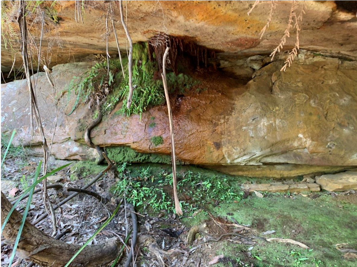
Photograph 5: View underneath undercut sandstone bed, water seepage observed
