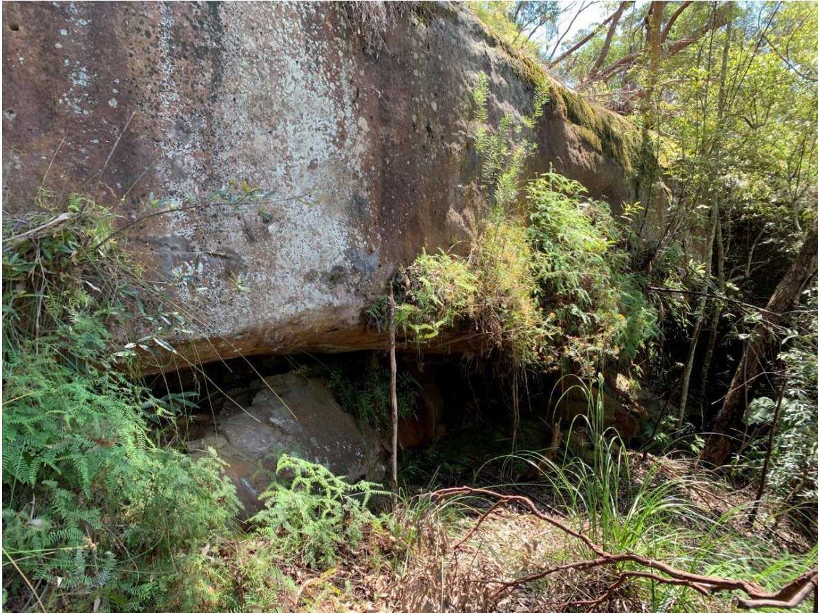
Photograph 3: View looking north-west, large sandstone bed with up to 2.5m undercut
