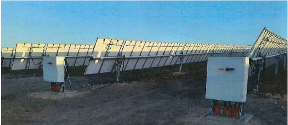
Figure 7 – Image of typical combiner boxes set at end of row of solar panels
