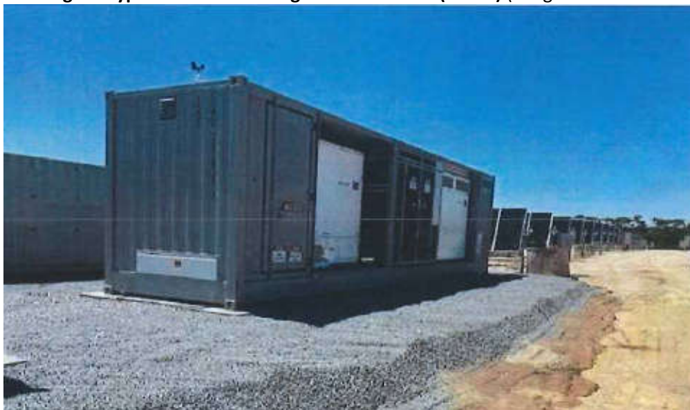
Figure 4 – Image of typical Medium Voltage Power Station (MVPS) (image taken from SEE)
